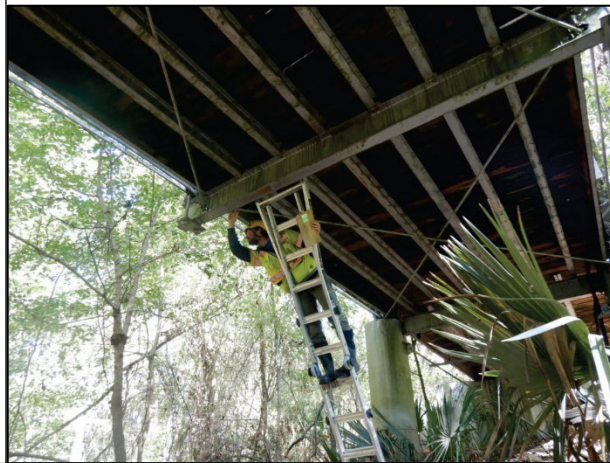
Hands-On Inspection of NSTM of the Iron Bridge at Tensas River National Wildlife Refuge, Louisiana
