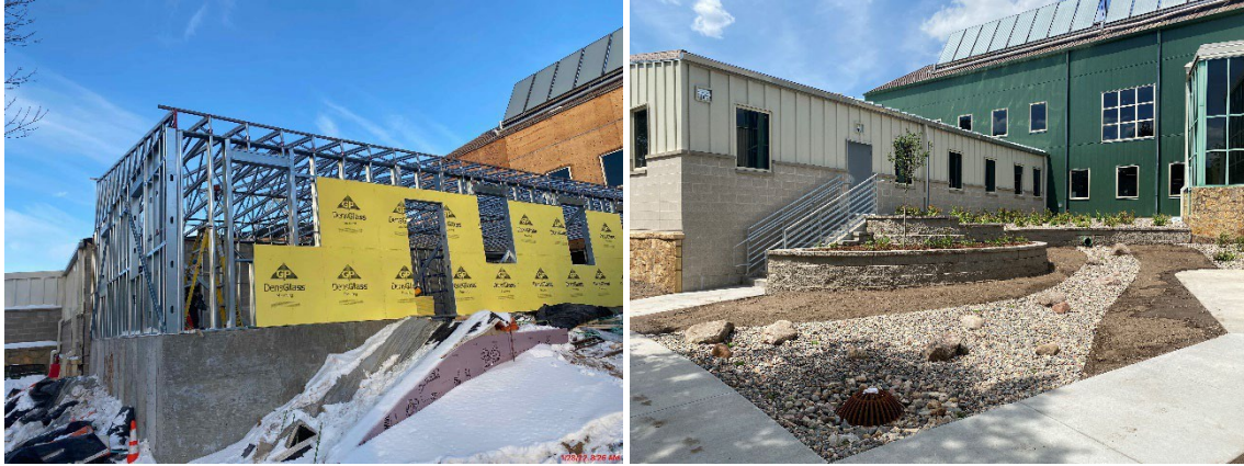
The Ecological Services addition to the MN Valley NWR, during construction and after completion.
